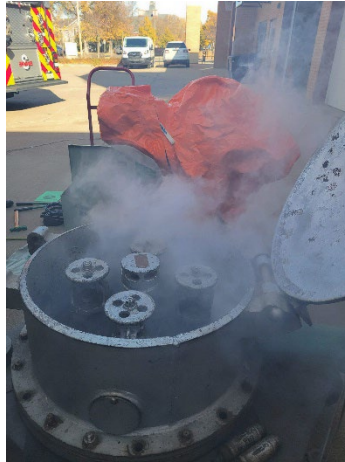
Above: Crewmembers contain a leak in a railcar “dome.”
